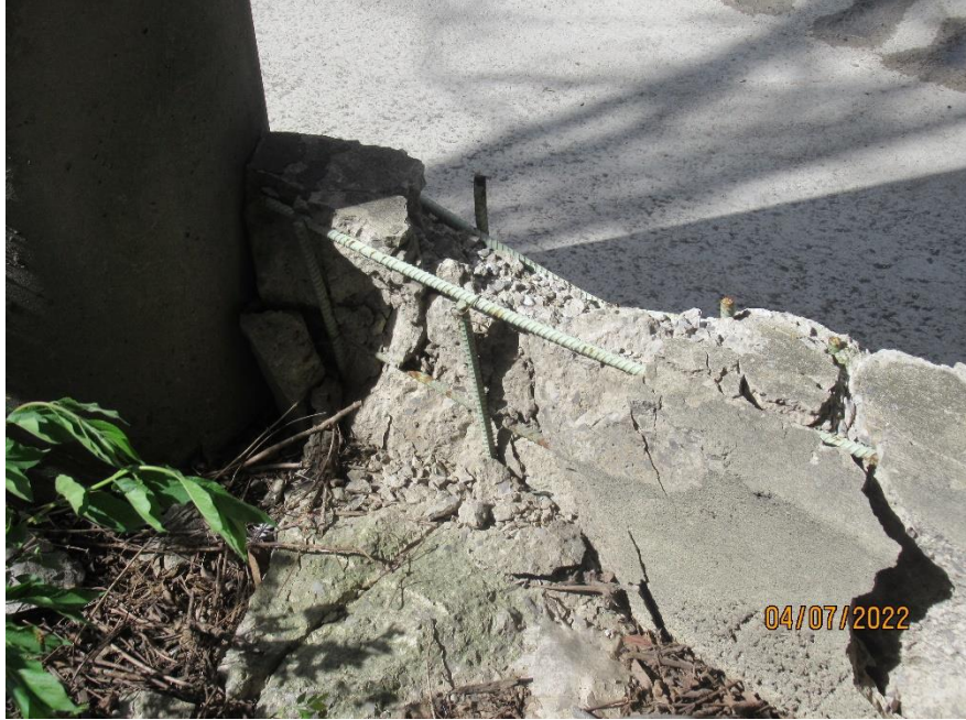
DAMAGE TO PARAPET - FROM BEAM REMOVAL – BENT #1
