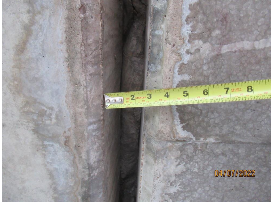
2.5" GAP BETWEEN BEAMS "B" AND "C" IN SPAN #4
