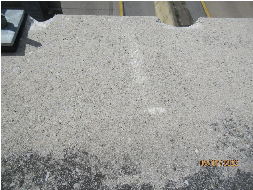
BACK OF SIGN - RIGHT CORNER - CRACK
