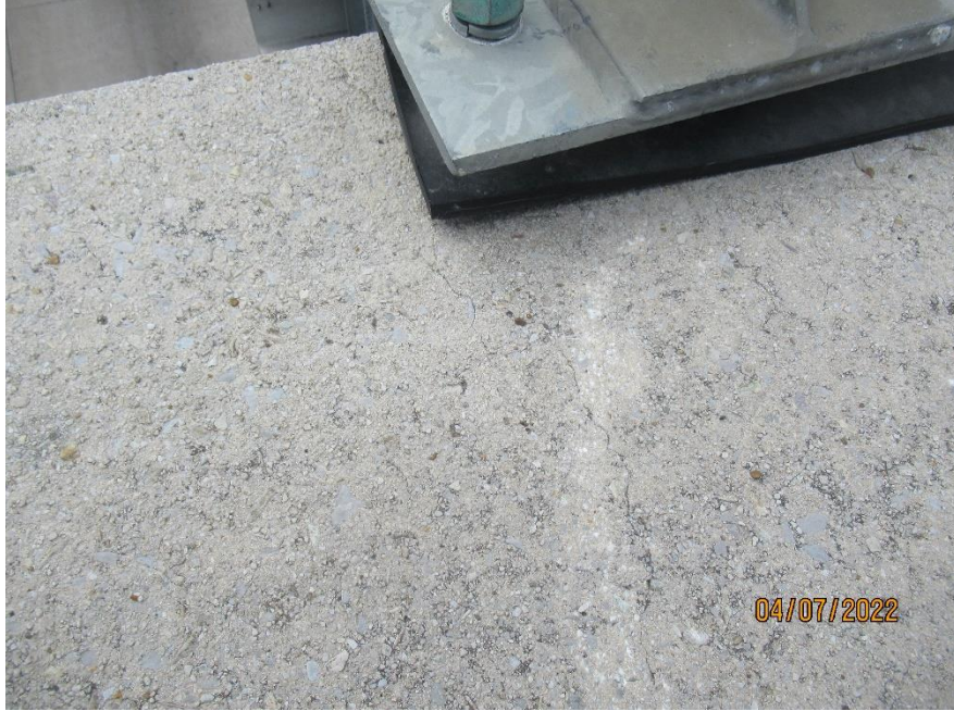
LEFT BACK OF SIGN – LEFT CORNER - CRACK
