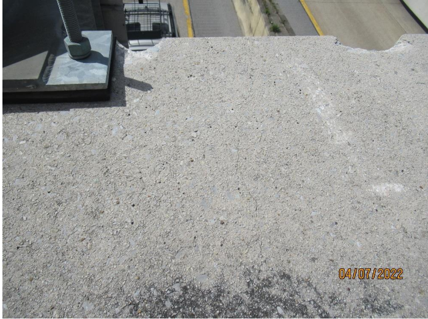
BACK OF SIGN - RIGHT CORNER - CRACK
