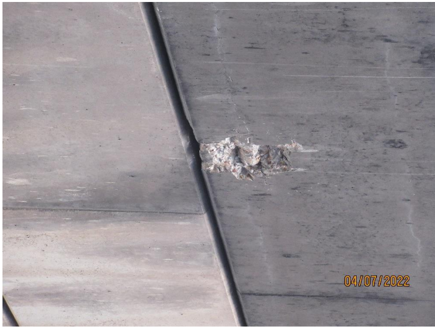
SPALLED BEAMS "P" AND "Q" - SPAN #2
