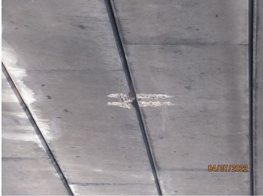
SPALLED BEAMS - "F" AND "G" - SPAN #2
