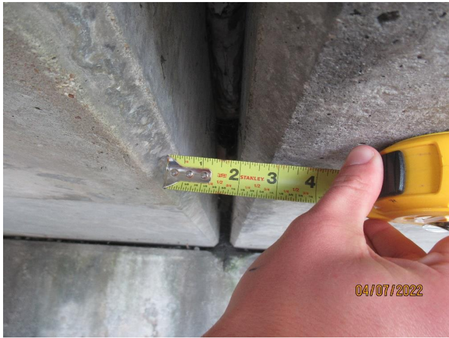
2" GAP BETWEEN BEAMS "A" AND "B" - SPAN #1
