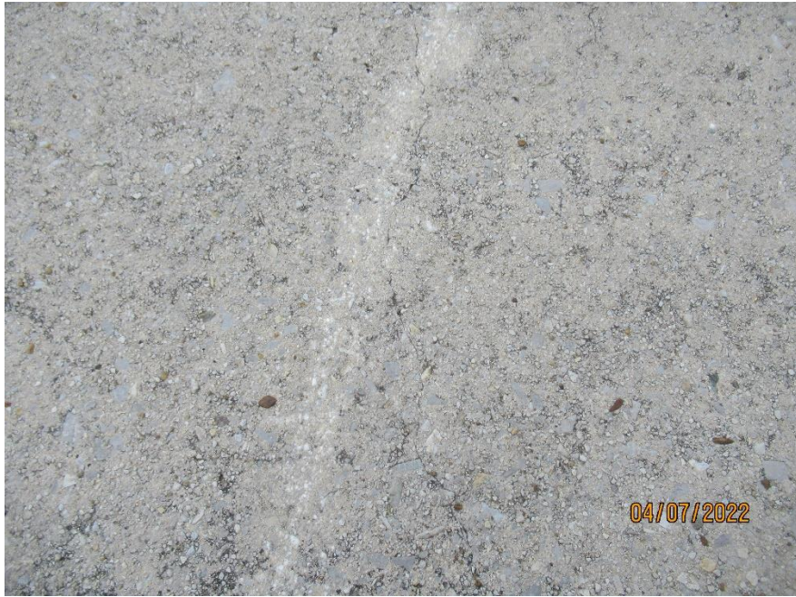
LEFT BACK OF SIGN – LEFT CORNER - CRACK
