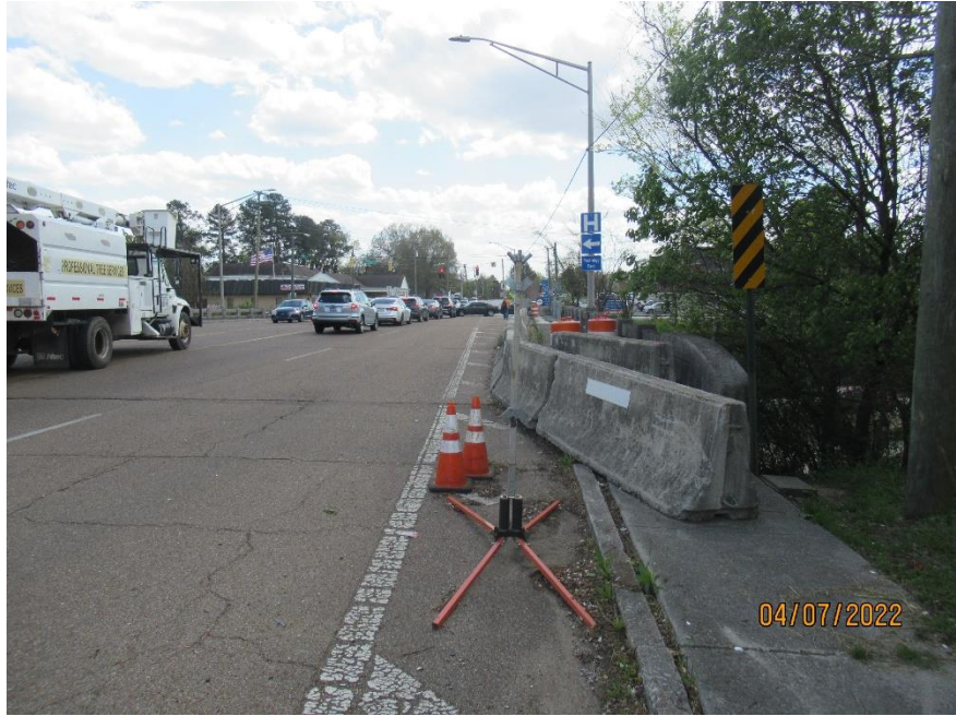
TRAFFIC CONTROL - LOOKING BACK - "SIDEWALK CLOSED" SIGN IS MISSING
